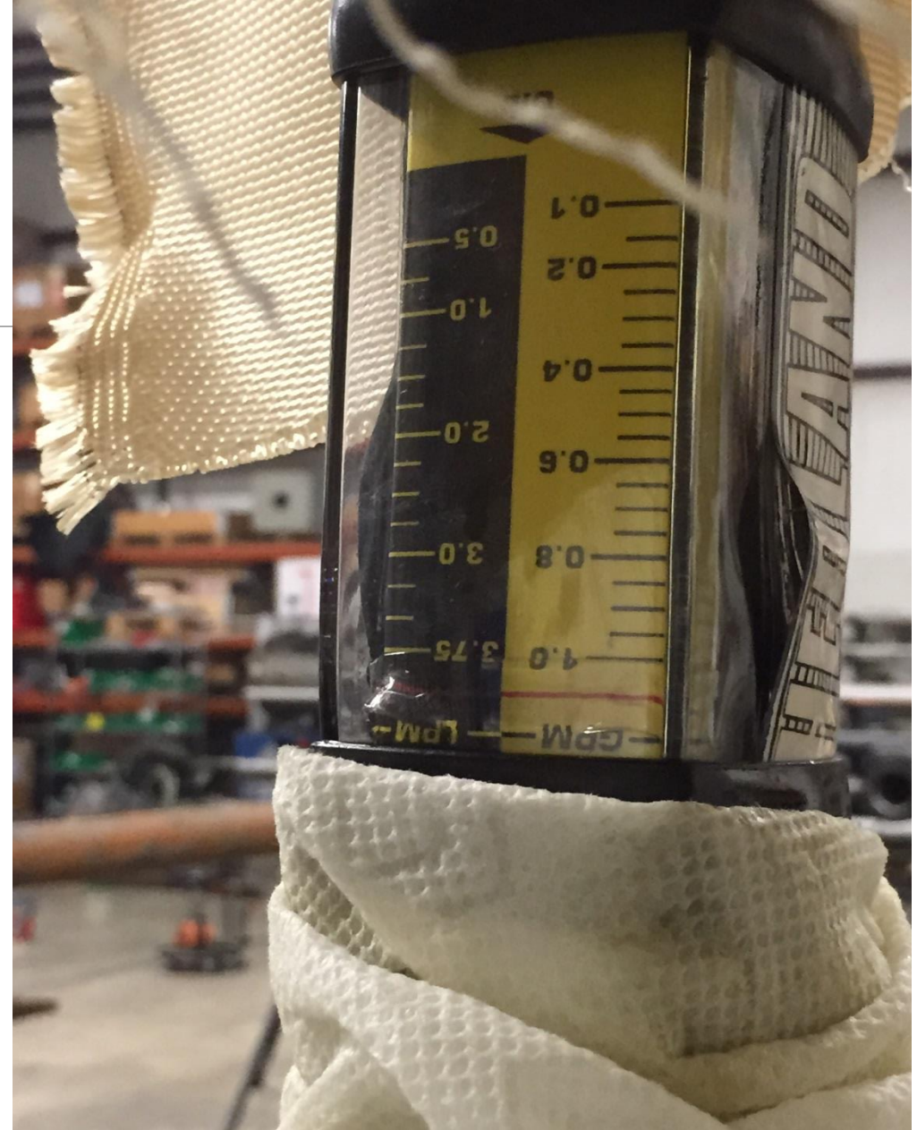
Figure 23. Damaged Flow Meter
